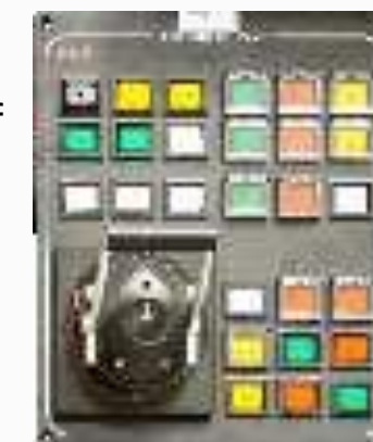
Control panel of full rotation remote control system
