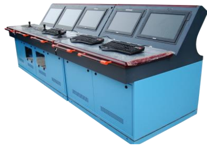
Engine control console
