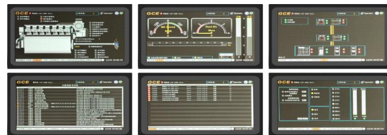
Low speed main engine remote control
