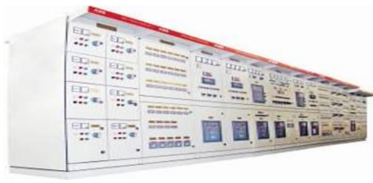
GCE Low voltage cabinet
